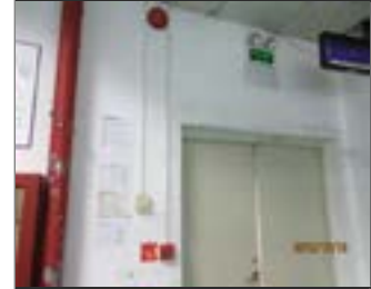
External photo(s) of the production unit(s) NO-23 Exit sign and emergency light and fire alarm.JPG
