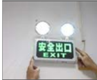
External photo(s) of the production unit(s) NO-25 Emergency light testing.JPG
