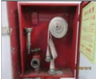
External photo(s) of the production unit(s) NO-27 Fire hydrant.JPG
