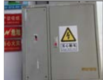
External photo(s) of the production unit(s) NO-18 Electricity box.JPG
