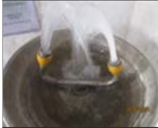
External photo(s) of the production unit(s) NO-21 Eye washing facility.JPG
