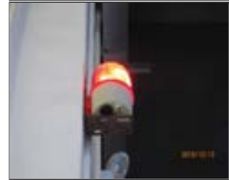
External photo(s) of the production unit(s) NO-26 Fire alarm testing.JPG
