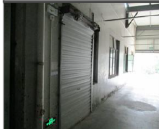
Photo of fire safety equipment The evacuation indicating signs and emergency lights along passageways.JPG
