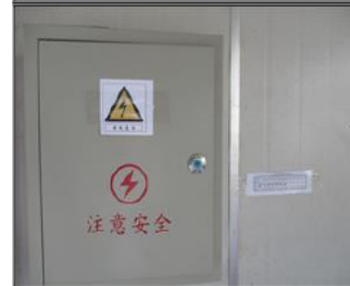
External photo(s) of the production unit(s) The warning signs for electricity.JPG
