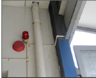
Photo of fire safety equipment The fire alarms.JPG
