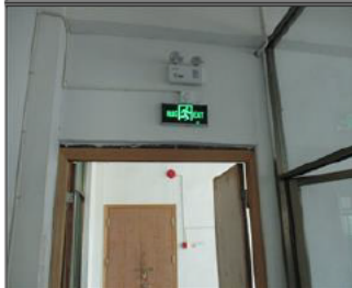
Photo of fire safety equipment The emergency exits with exit signs and emergency lights.JPG
