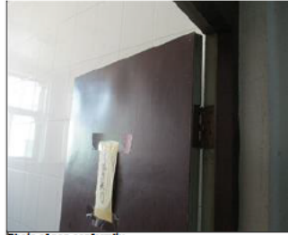
Photo of non conformity NC Toilets were not identified with genders and no basic supplies.JPG
