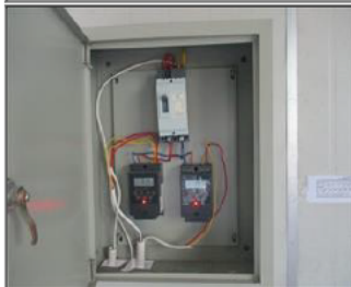
Photo of non conformity NC No inner protective covers and outer protective covers were not locked.JPG
