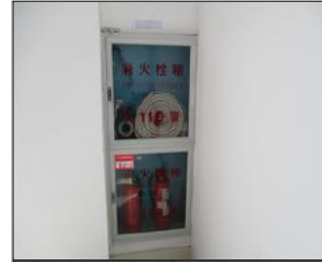
Photo of fire safety equipment The fire fighting equipment.JPG
