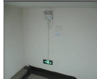
Photo of fire safety equipment The evacuation indicating signs and emergency lights along stairs.JPG
