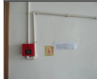
Photo of fire safety equipment The buttons for fire alarms.JPG
