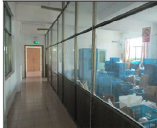
Photo of non conformity NC No evacuation plans at production areas.JPG
