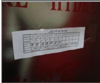
Photo of fire safety equipment The inspection records for fire hydrants.JPG
