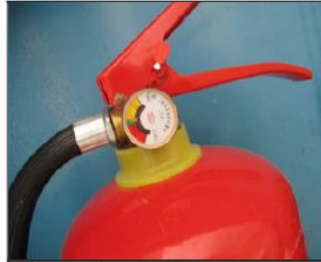
Photo of fire safety equipment The fire extinguishers were in good condition.JPG
