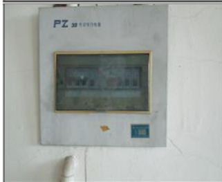
Photo of non conformity NC 5 electric switches missed function labels as warning signs.JPG
