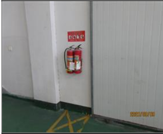
Photo of fire safety equipment 3. Fire extinguishers.JPG
