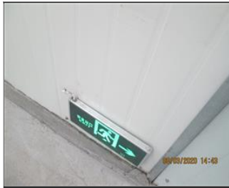
Photo of fire safety equipment Evacuation signs.JPG
