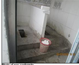
Photo of non-conformity the hygiene of toilet was not maintained well and no private doors were installed in dormitory toilet.JPG
