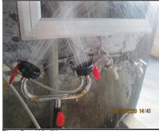
Photo first aid facilities Eye washing facilities.JPG
