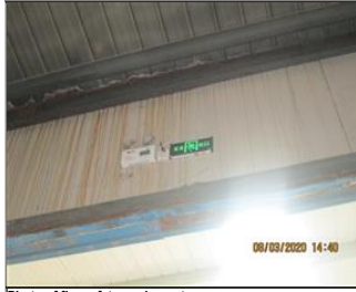
Photo of fire safety equipment Emergency sign.JPG
