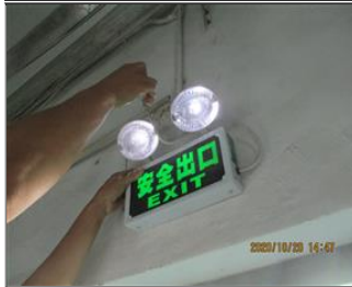
Photo of fire safety equipment Fire emergency lighting testing.JPG
