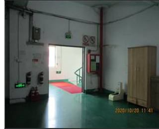
Photo of fire safety equipment Fire facilities 2.JPG
