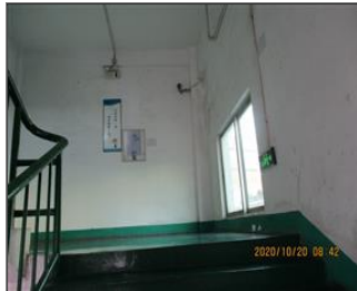
Photo of fire safety equipment Fire stairs.JPG
