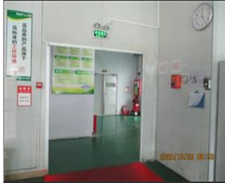
Photo of fire safety equipment Fire exits.JPG
