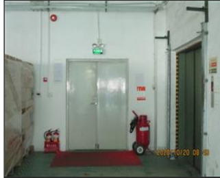
Photo of fire safety equipment Fire facilities 1.JPG
