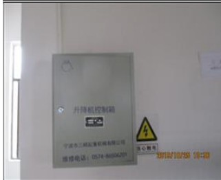
Photo of the inside of the main production hall Electric box.JPG
