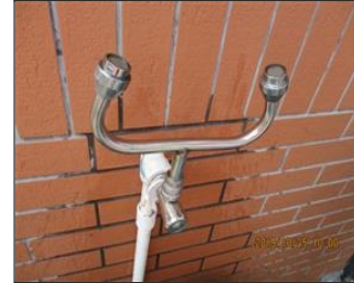
Photo first aid facilities Eye washing station.JPG
