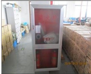
Photo of fire safety equipment Fire extinguisher and fire hydrant.JPG
