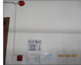
Photo of fire safety equipment Fire alarm.JPG
